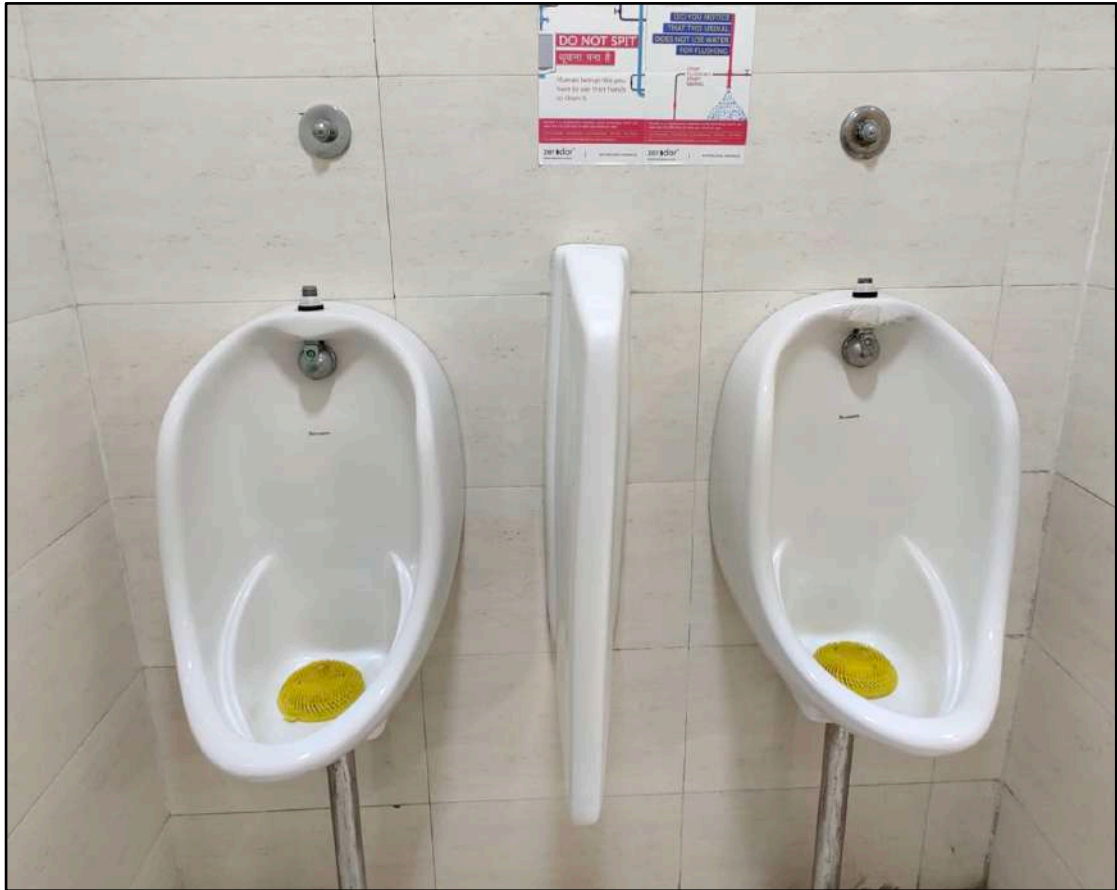
Waterless urinals in the staff room helps conserve water
