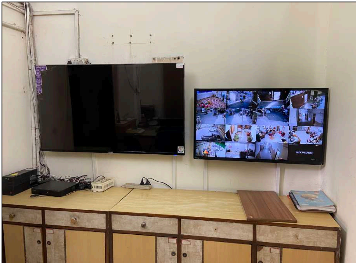
Revamped CCTV system for security and surveillance in the college
