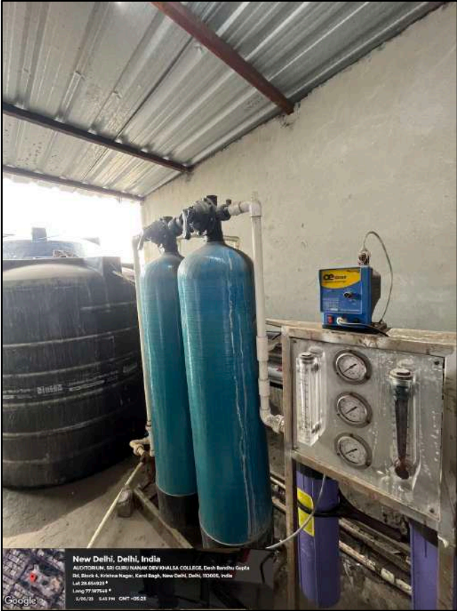
Water Treatment Plant in the college
