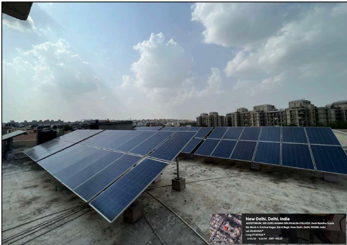
Rooftop Solar panels for generating electricity through a renewable source
