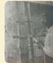
Identifying the fatal low-height brackets on Telephone - Post
